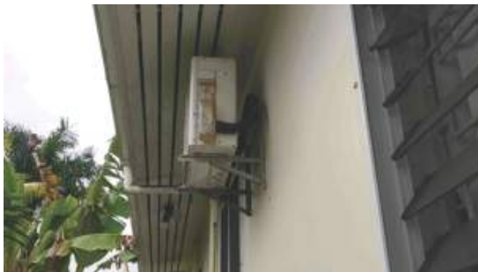
Figure 15: North-Facing A/C Condenser In Fiji Shaded By Overhang And Trees
