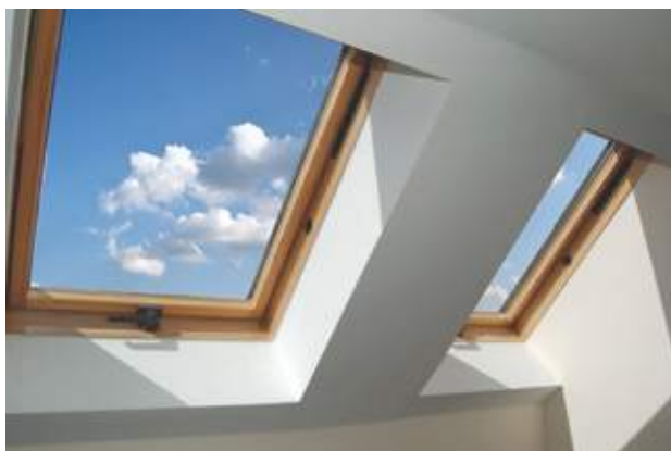
Figure 2: An Example Of Incorrectly Placed Skylights Facing East
